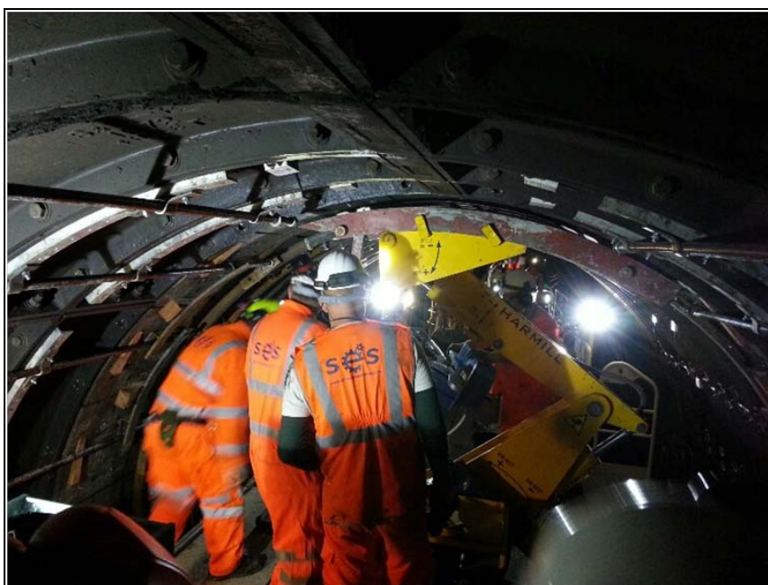
Cutting head being readied to begin removal of crown section of expanded concrete ring.
