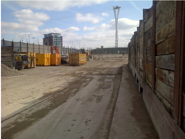
Figure 6-5 The majority of the predominantly industrial use Silvertown site is formed of hard standing.
