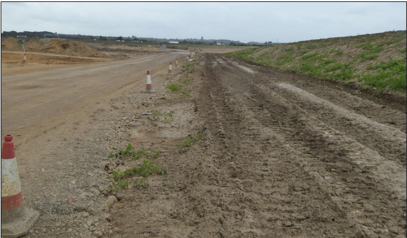
Figure 3-3 Mechanically stabilised soil (left of cones) and unbound soil (right of cones)
