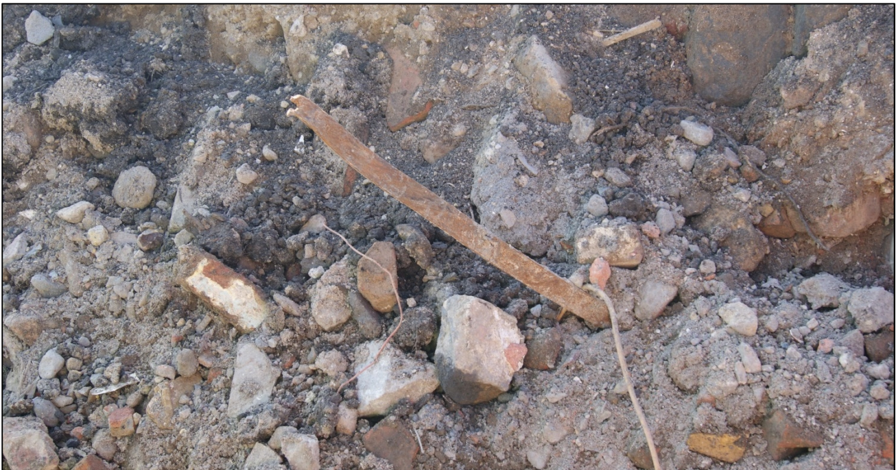
Figure 3-7 Loose material, including metal bar, present at edge of haul road
