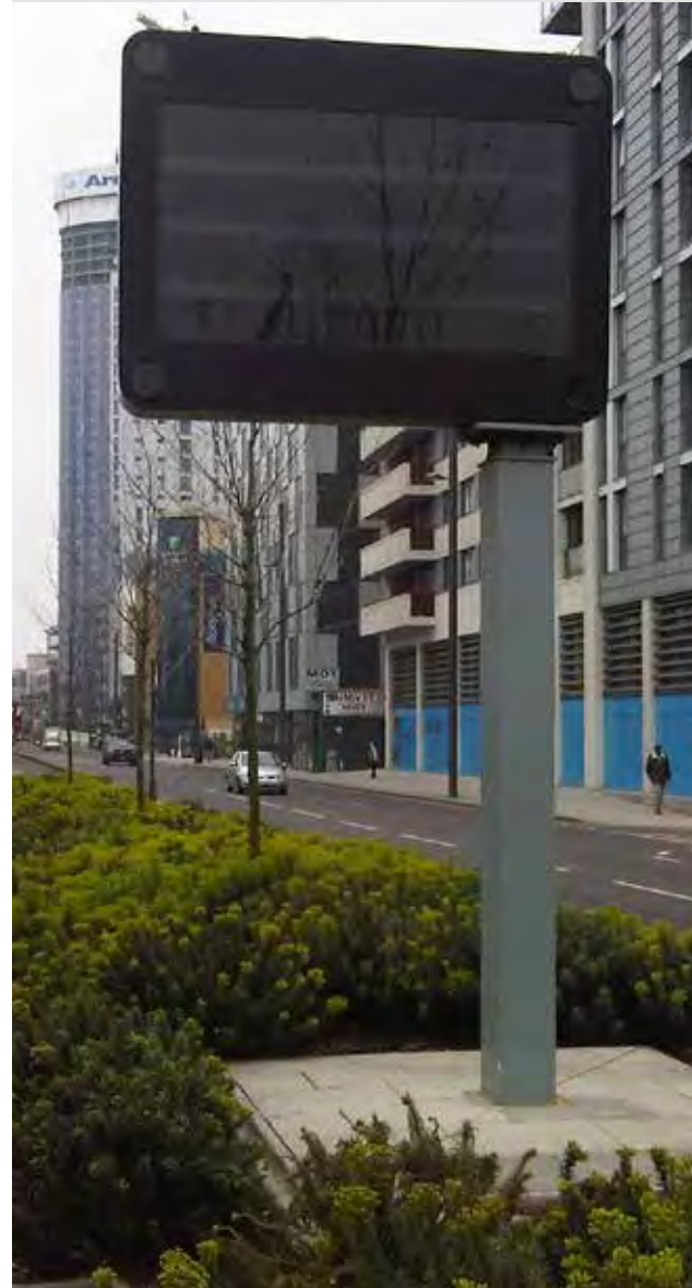
Figure 260: Variable message sign (VMS) when not in use
