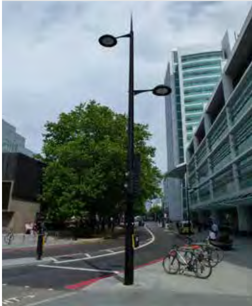
Figure 282: Highway lighting column illuminating footway and carriageway
