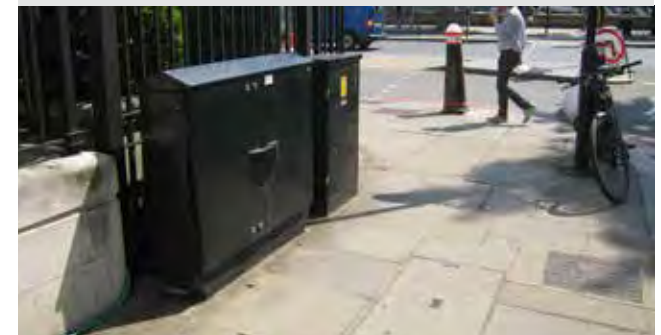
Figure 258: Utility boxes placed at the back of the footway
