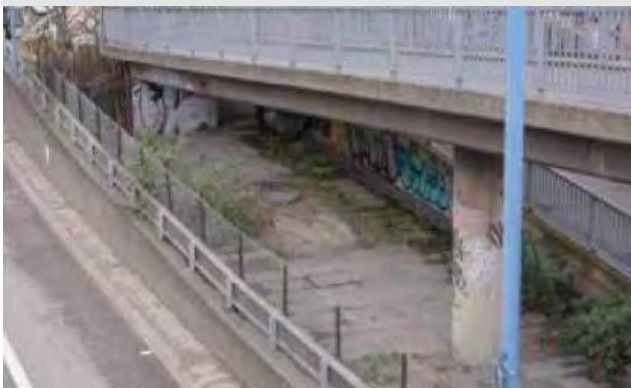
Figure 29 I: Spaces on the network which appear to be uncared for should be targeted for reinvigation
