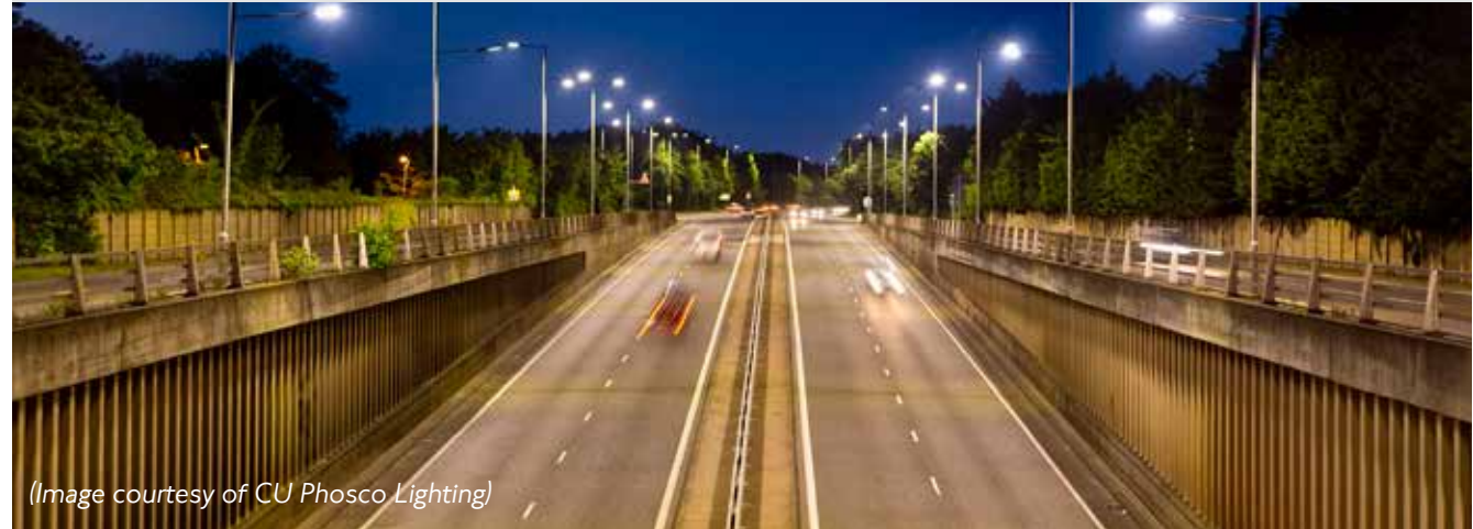
Figure 283: LED lighting recently installed
