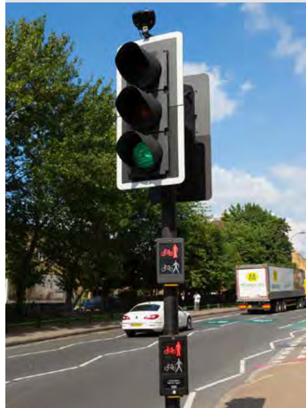
Figure 158: Traffic signal for toucan crossing
