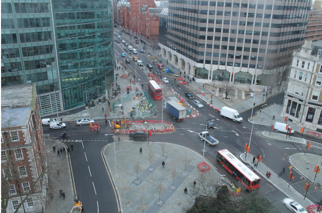
Simplifying traffic movements to create space for pedestrians and cyclists at Holborn Circus
