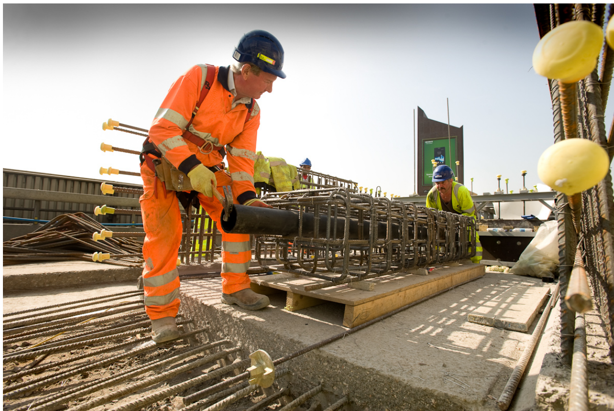
Hammersmith Flyover – finding ways to deliver complex infrastructure projects quicker, better, simpler and cheaper
